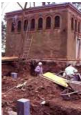
► Photograph of the construction site of the Korean Pavilion, 1994. ©Mancuso e Serena Architetti Associati. Courtesy of ARKO Arts Archive, Arts Council Korea.
